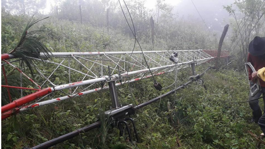
Downed Transmission Tower for Radio Progreso
